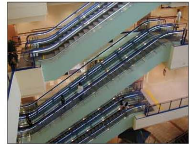
Light Under Handrail
