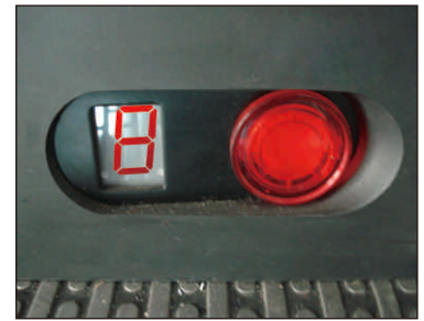
Fault Display for S and F Type
